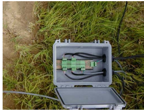
Smart interface connected to DataBus, which is connected to Smart Datalogger
