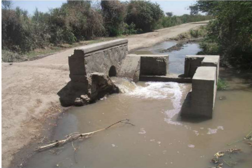
Flow division structure with missing control gates at Meki Ziwai irrigation scheme
